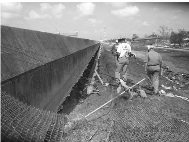
Fig. 11. Eroded trench at the rear (inboard) side of the floodwall at the south end of the south breach at the east bank of the IHNC at the west end of the Lower Ninth Ward
