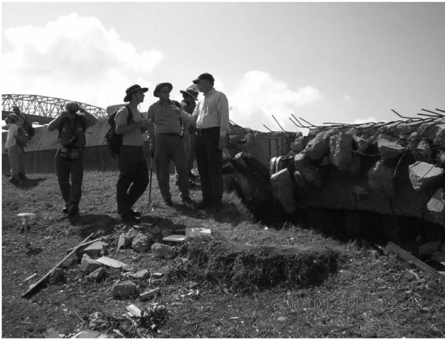
Fig. 10. Close-up view of crushed (impacted) concrete floodwall at the south end of the south breach at the east bank of the IHNC at the west end of the Lower Ninth Ward
