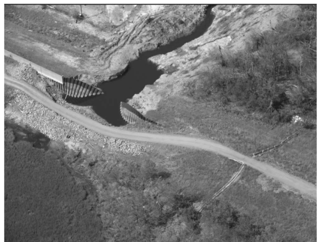
Fig. 3. An example of one of the numerous failures (breaches) that occurred at “transitions” between disparate, adjoining flood system elements. (From left to right: concrete floodwall, sheet pile wall, and earthen levee.)
